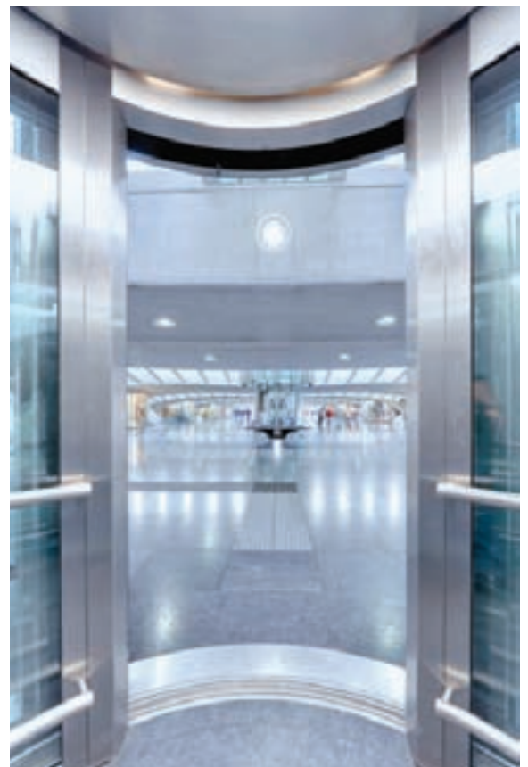
Photo right, above: Dramatic lighting accents these Schindler escalators that carry passengers to and from the track level of the station. Photo right, bottom: A Schindler elevator opens to the station's upper level.
