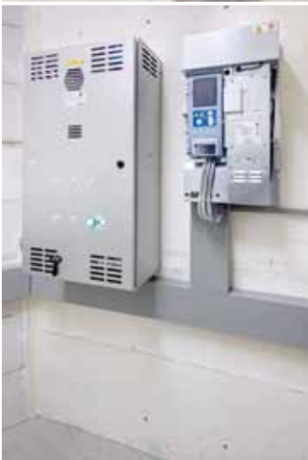
Controller and frequency converter
