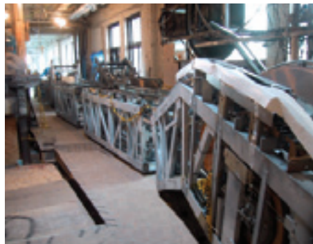
Photo right: Hoisted in modules to the 67th floor, all Schindler escalator sections are aligned for assembly and installation. Photo below: Passengers enjoy a historical video of Rockefeller Plaza projected onto the dome of the sky shuttle elevator car as it travels to the Top of the Rock observation deck.
