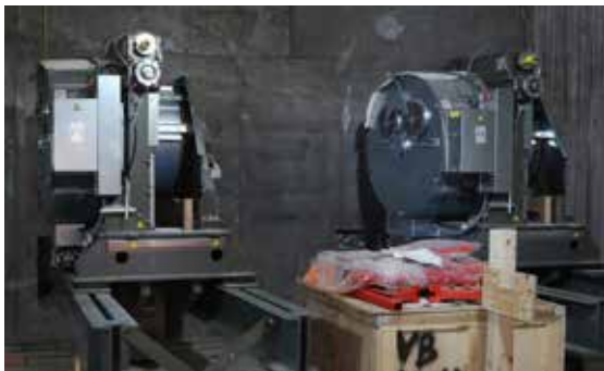
560 machines in a low-rise machine room
