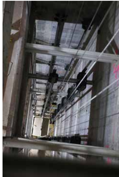
Looking down into the hoistway; the top of the false car is in view.
