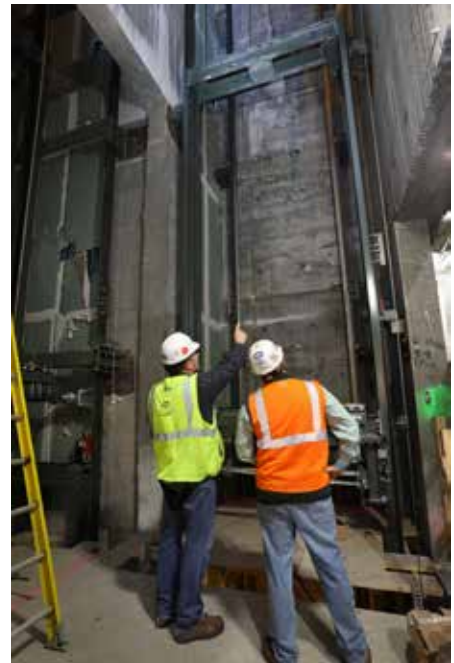
(l-r) Dineen and Jackson look at an installed service car frame and platform.
