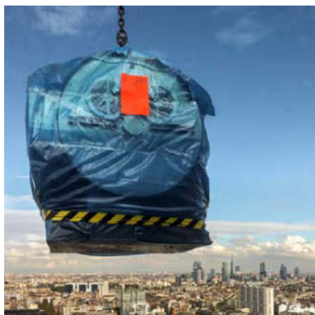
One of the high-performance motors for the Libeskind Tower is lifted by crane.
