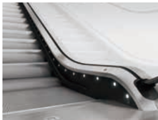
Skirt lighting, spots
