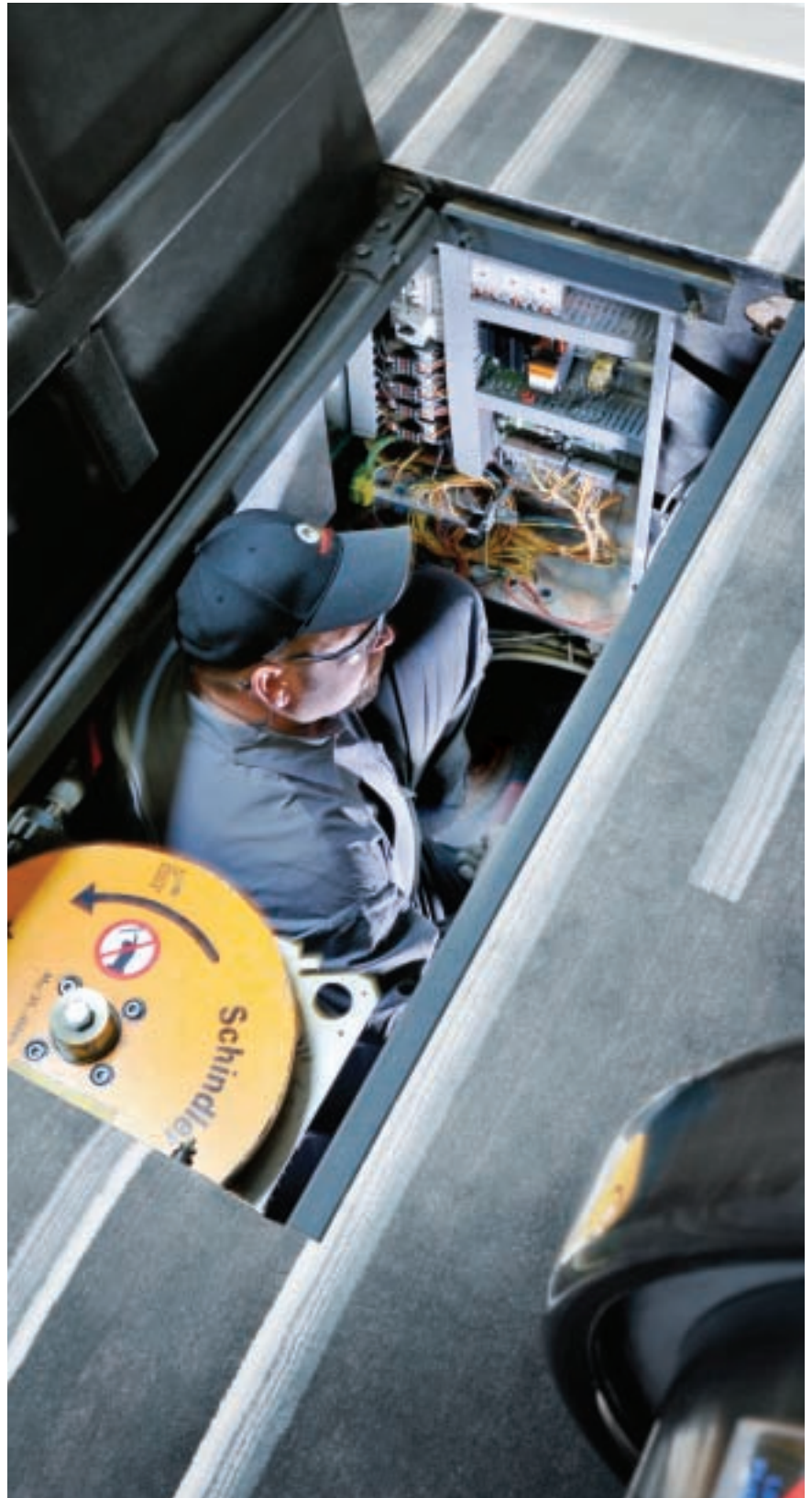
A Schindler technician makes final adjustments to an escalator’s new solid state controller.
