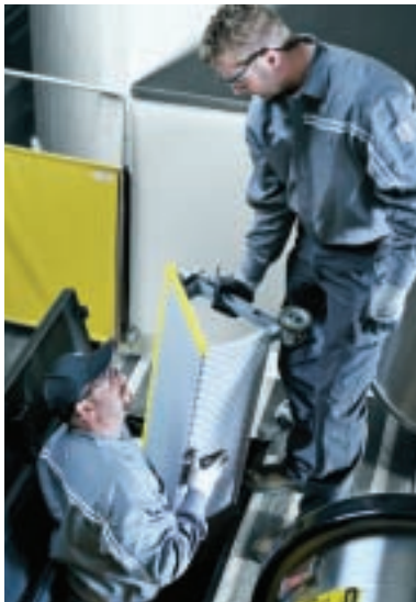
Photo above: Schindler technicians install new steps as part of an escalator upgrade. Photo right: Fully upgraded escalators can look and perform like new at lower cost and with less inconvenience.
